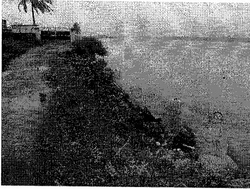
a. Eroding road leading to the entry gate of the proposed port
